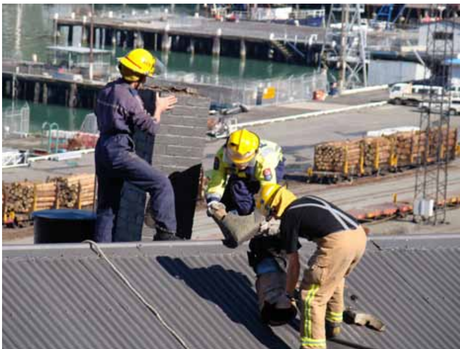
Members of Lyttelton's Volunteer Fire Brigade fixing one of the chimneys damaged during the September 2010 earthquake
